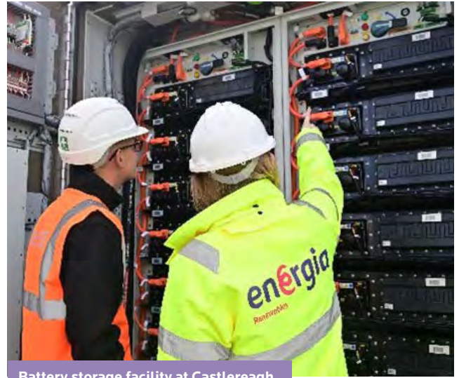
Battery storage facility at Castlereaigh
